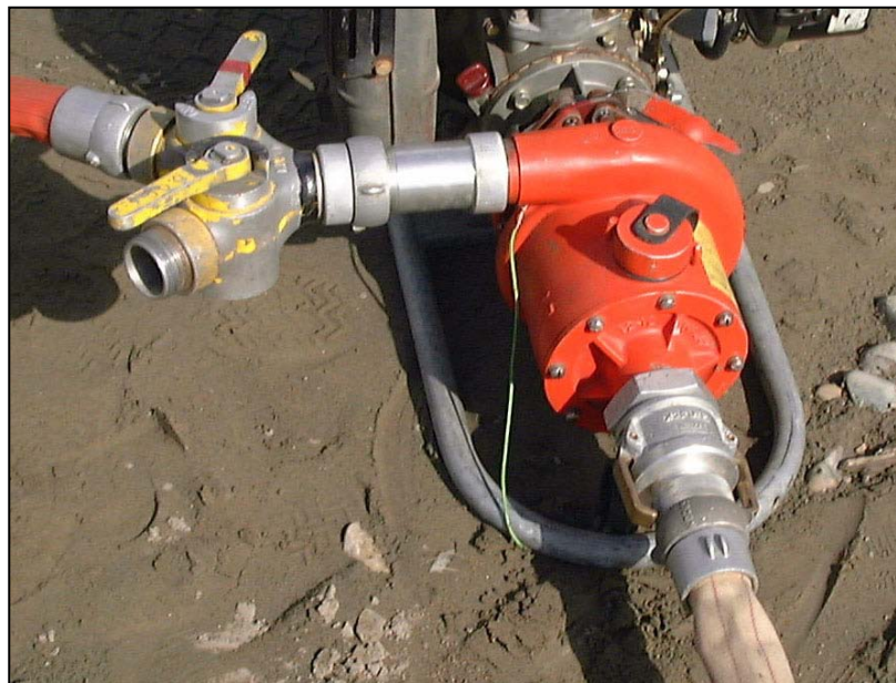
Figure 4.10 – Wajax in a closed relay being fed via a relay adaptor
