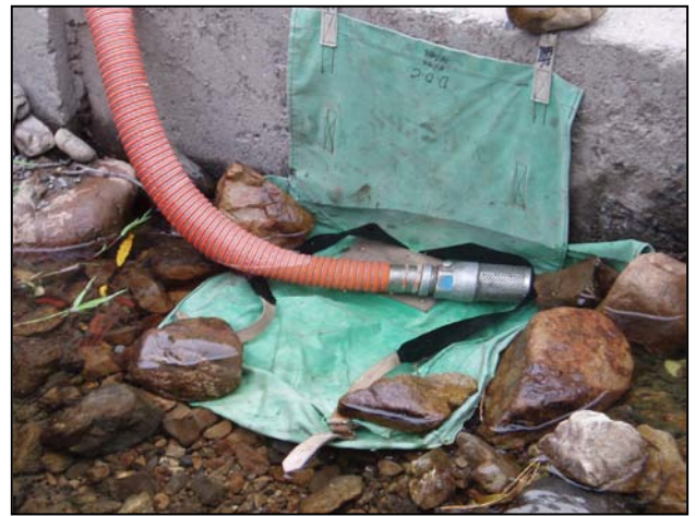
Figure 2.5 – A hose pack used to minimise clogging of a suction strainer
