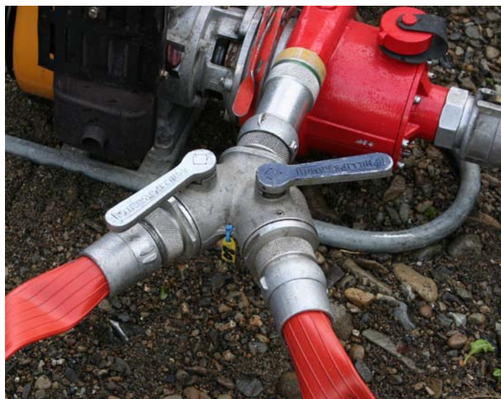
Figure 4.4 – Controlled dividing breeching connected on the pump outlet
