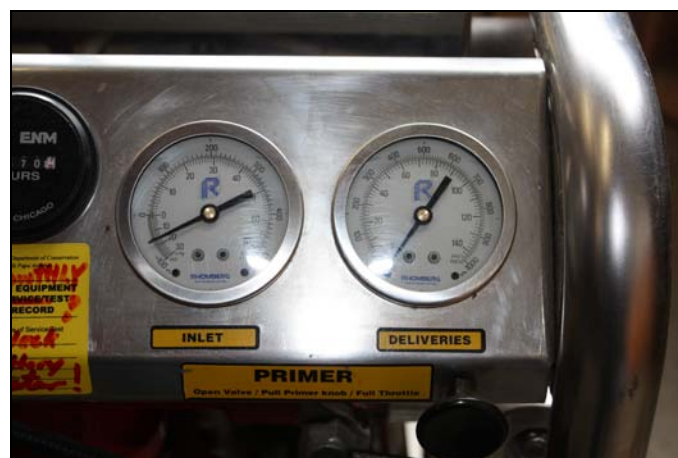
Figure 2.3 – Pumps with gauges
